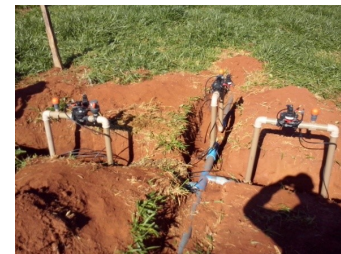
Fig. 8. Automatic irrigation valves installed in the rural property. The valves receive the opening and closing instructions from the system through the solenoid relays.
